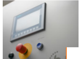
Digital control panel
