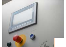
Digital control panel
